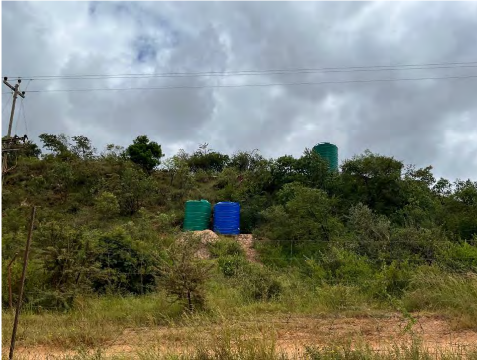
Photo 1 : Water storage tanks and power supply on Happy Valley Claim
